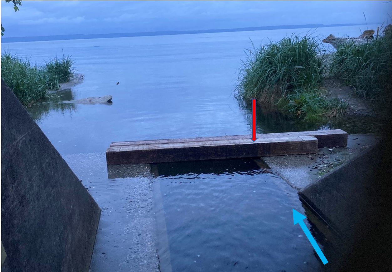
Figure 2. Outlet of the backwatered Lund's Gulch Creek culvert (under BNSF railroad) at high tide May 17, 2022 (11.00 ft. MLLW, 5:14 AM). Puget Sound is in background. Stream flow direction is shown with blue arrow. The red arrow shows the location of the downstream staff gauge, also shown in Figure 3.
