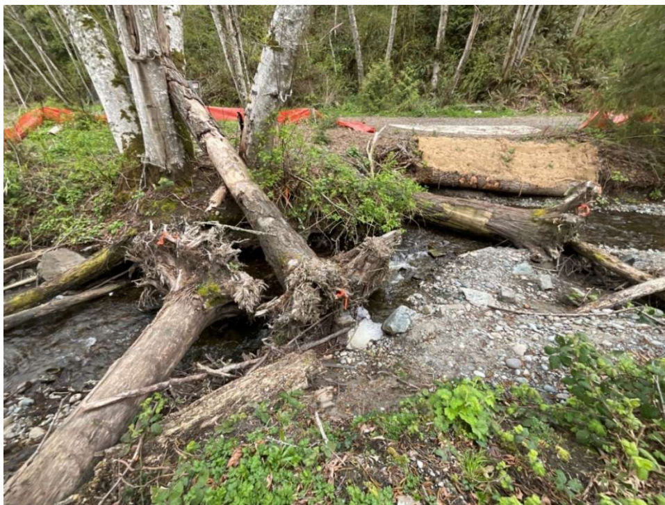
Figure 16. Large Woody Material (flagged) with Rootwads Placed in Lund's Gulch Creek Segment 3
